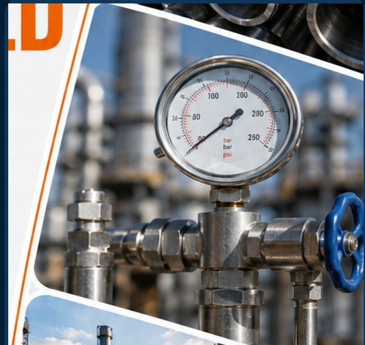
Fittings, valves, and pressure lines
